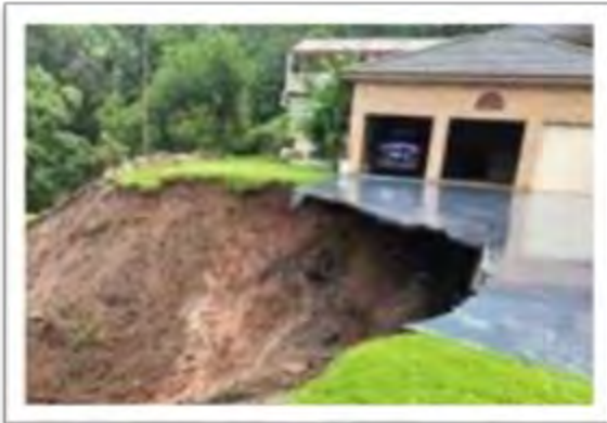
Housing / Local govt., erosion and stability
